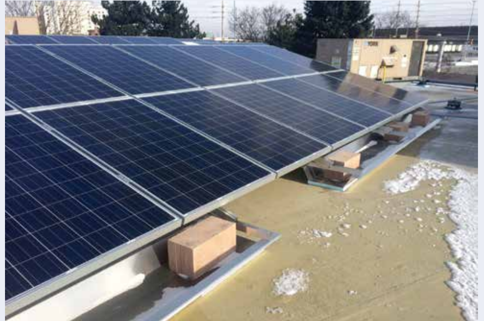
Desjardines Financial The main roof of this high-profile project in downtown Mississauga is 10,000 square feet. “The owner wanted Kemper System and a long-term warranty,” says Hunter, who specified full roof waterproofing with the KEMPEROL® 2K-PUR reinforced resin membrane system. A solar array was installed on the roof using platform supports. Contractor: Triumph Inc. (Toronto)
