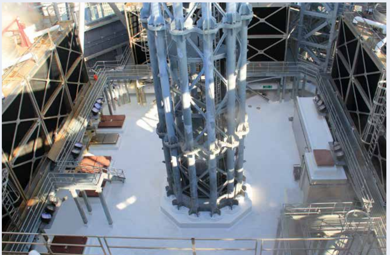
The square area at the base of the spire is surrounded by a three-story framework for mechanical equipment inside the communications platform ring.
