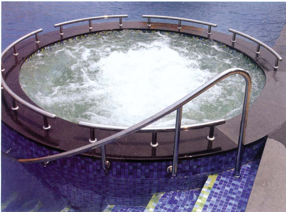
Jacuzzi in operation at the water resort.
