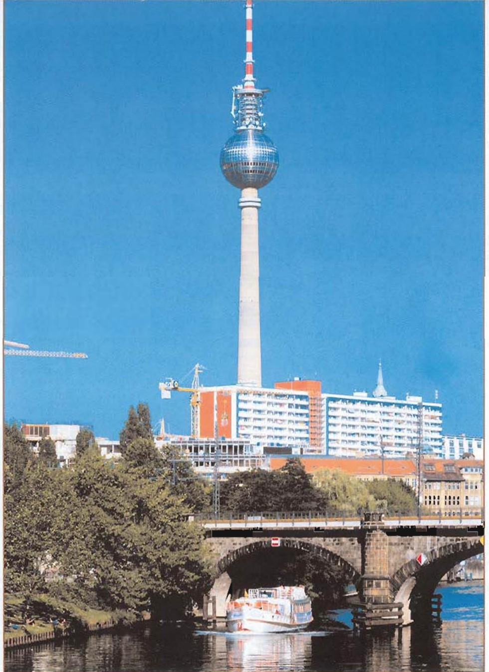
Alexanderplatz, the Berlin television tower built in 1969, presented waterproofing challenges. A strong bond was necessary between old concrete and repair mortar.
